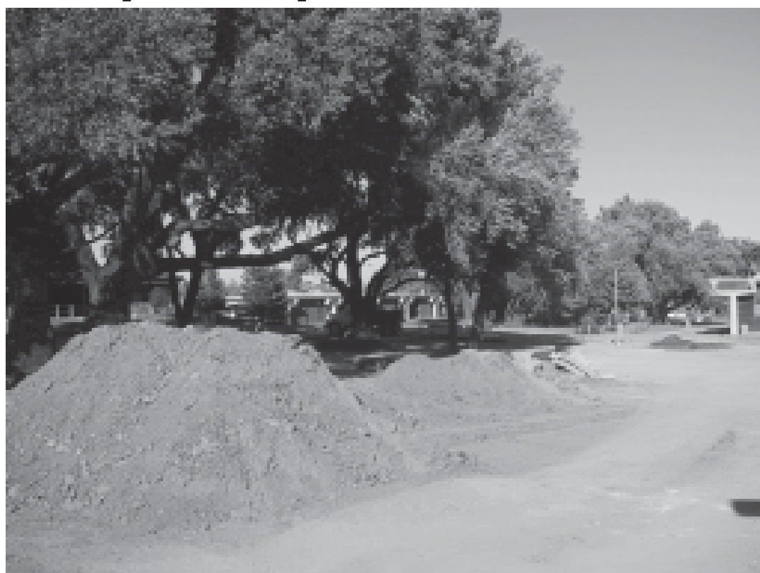
Over the summer, the San Marin campus was torn up to allow for replacement of heating/air conditioning systems, phones and PA. But when students returned to school on August 26, the campus the piles of dirt were gone and the classrooms, for the most part, were cool.
